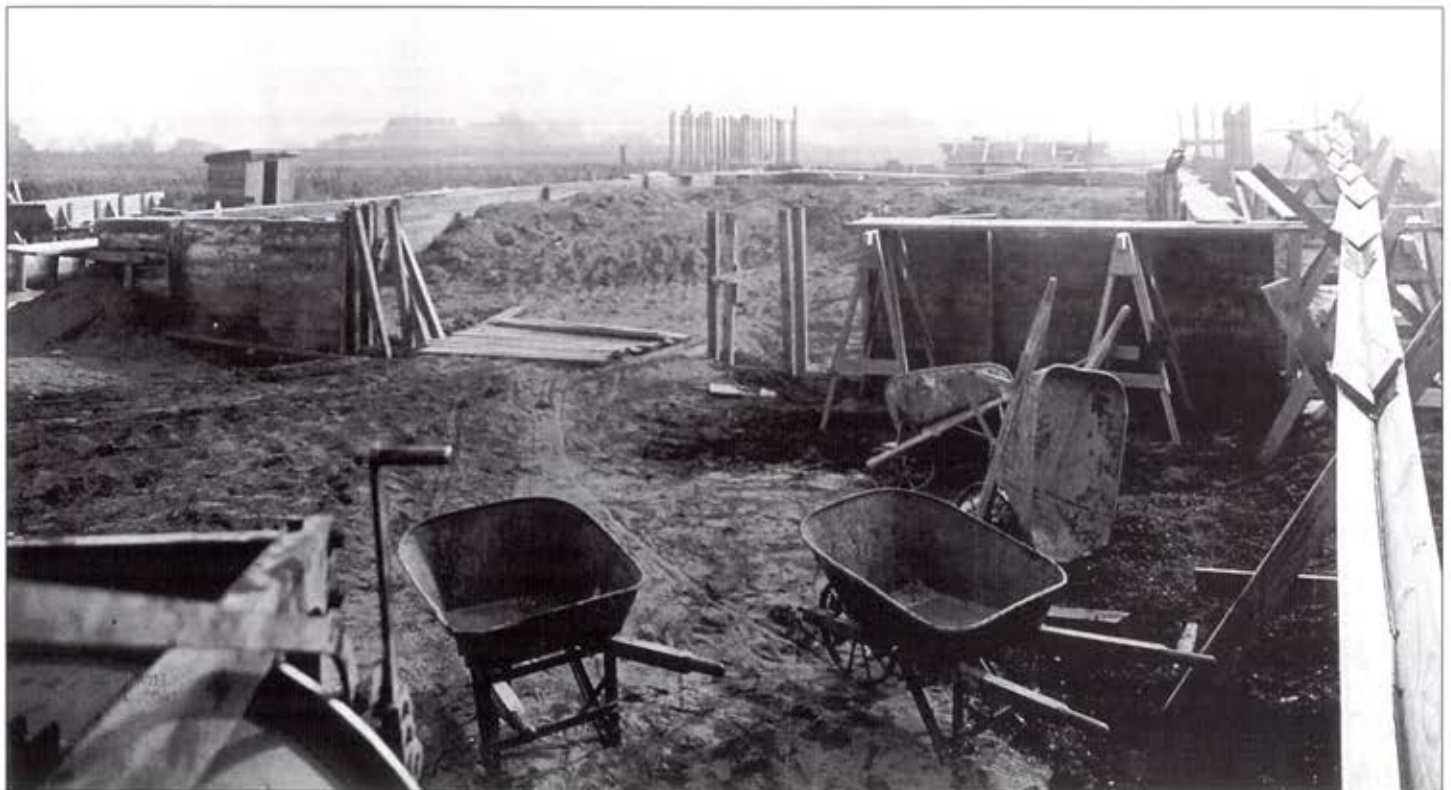
▲ Construction of the Dempster Station was well chronicled by photographers. Foundation work was well underway on October 30, 1924.—Illinois Railway Museum Collection via J. J. Sedelmaier Productions Collection
