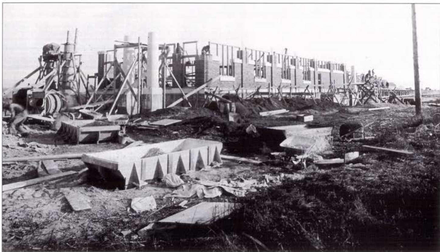
▲ In this view taken on November 20, 1924, masonry work continues, platform construction can be seen at the far right, and the pillars at the front entrance have begun to appear.—Illinois Railway Museum Collection via J. J. Sedelmaier Productions Collection
